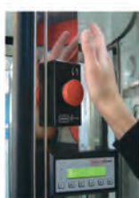
EMERGENCY PUSH BUTTON
