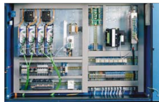
Electrical cabinet Open and easily surveyed panel includes digital control, cooling fan, transformers and control.
