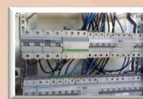
REVISION INST. ELECTRICA BT
