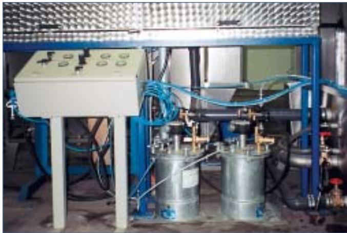
Pressure tanks and control cabinet for automatic application of separating agent for profiles
