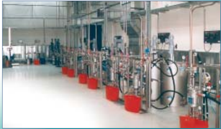
Colour mixing tanks in the automotive industry
