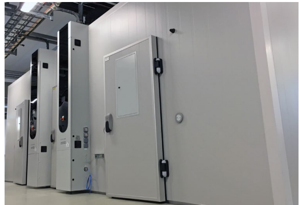
SET OF 10 FITOCLIMA 25.000 HP GROWTH ROOMS AT AGRICULTURE RESEARCH CENTER
