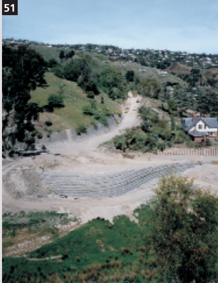
51. Retaining structure with Terramesh® S for new residential area, Christchurch, -New Zealand.
